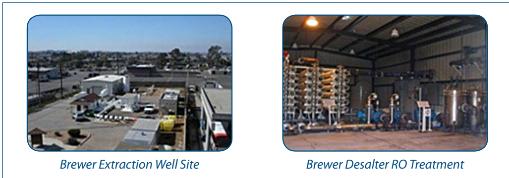
Figure 10-4: Brewer Desalter Facility Equipment
