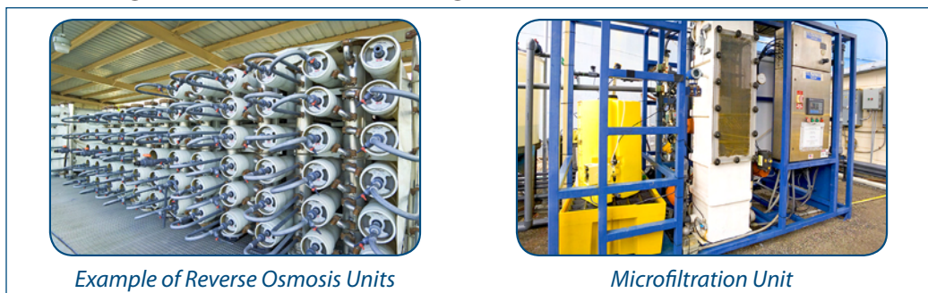
Figure 10-2: Treatment Technologies Used at West Basin’s Pilot Plant
